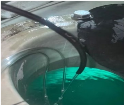
Instrument Drainage Pipeline
