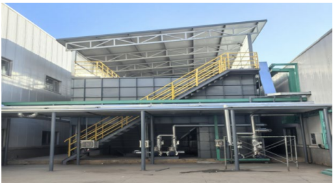
Operation of the Advanced Fluoride Removal System
